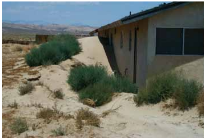
Figure 13: Rancho Seco residence has sand accumulation on the upwind side of the house.
