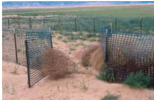
Figure 9: Porous wind fences are commercially available. They trap blowing tumbleweeds as well as sand. In areas with endangered species, such as the desert tortoise, openings should be provided at intervals to allow for continued natural migration of the animals.
